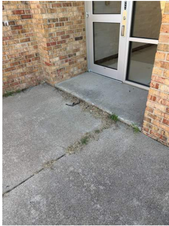
PHOTO 7 - NON-ADA COMPLIANT STOOP
