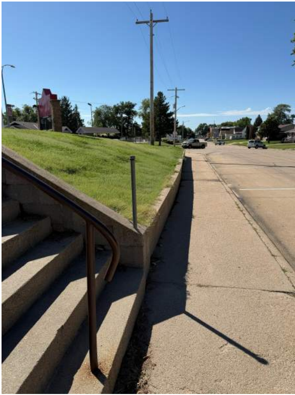
PHOTO 6 - LEANING RETAINING WALL
