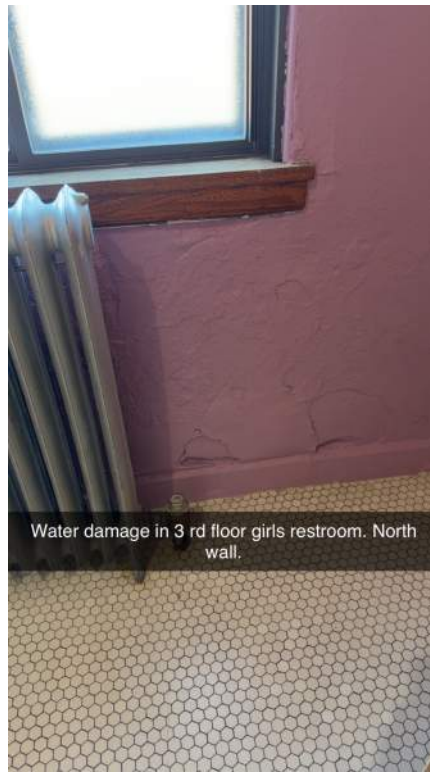
PHOTO 9 - WATER DAMAGE @ NORTH WALL
