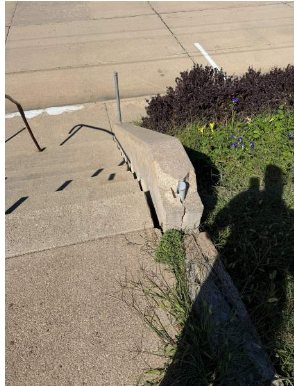
PHOTO 5 - DAMAGED STAIRS/ RAILINGS
